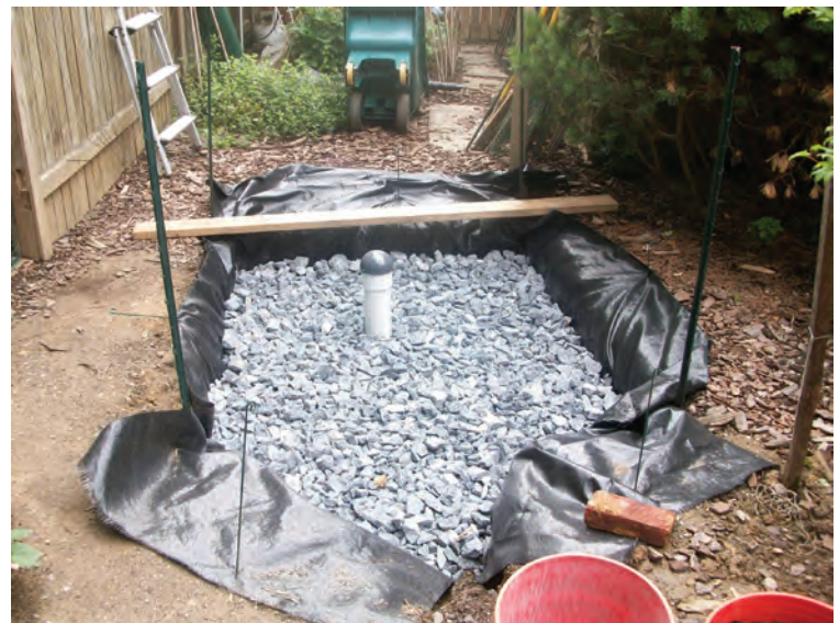
Figure 4.5. Dry Well installation with an observation well, shown after gravel is placed, before pea gravel (Source: Lancaster County Conservancy - Urban Greening Program)
