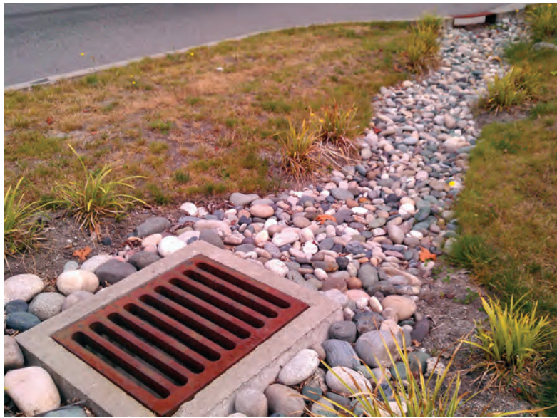
Roadside Infiltration Trench (Source: Flickr Creative Commons, Wendy Cutler)
