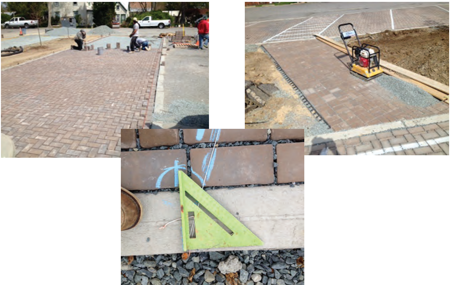
Figure 3.10. Installation of pavers (top left), compaction (top right), and filling spaces with pea gravel (bottom).
