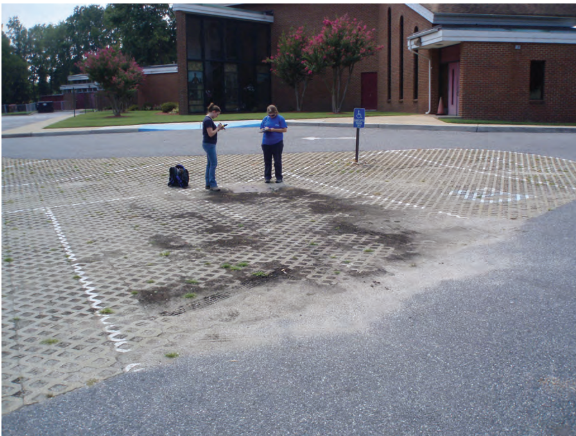
Figure 3.6. Permeable paver installation without pretreatment or filtering. Clogging evident from sediment and grit from adjacent surfaces.
