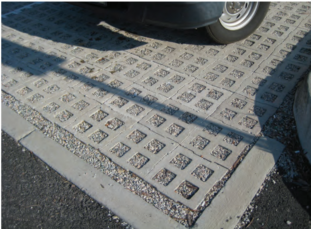
Figure 3.3. Permeable paver parking installation, light commercial scale. (Source: New York State Stormwater Green Infrastructure)
