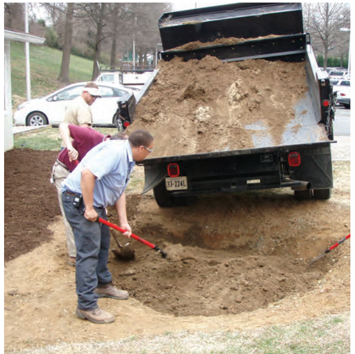
Figure 2.14. Add soil mix into excavated area until it reaches desired elevation for Rain Garden surface.
