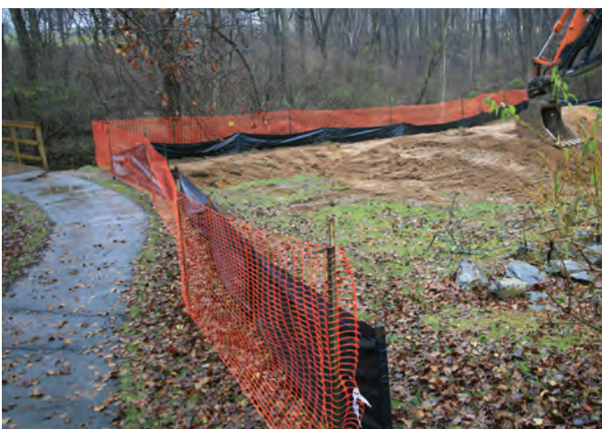
Figure 2.10. Install silt fence below the Rain Garden construction site for erosion and sediment control.
